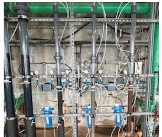
CDM Smith partnered with SGWASA to conduct the PFAS Mitigation Program.
